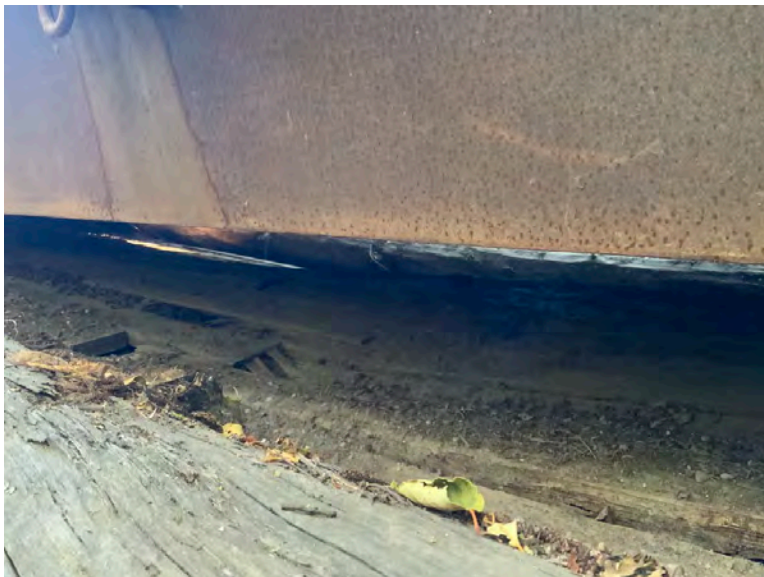
Old log bridge collapsing
